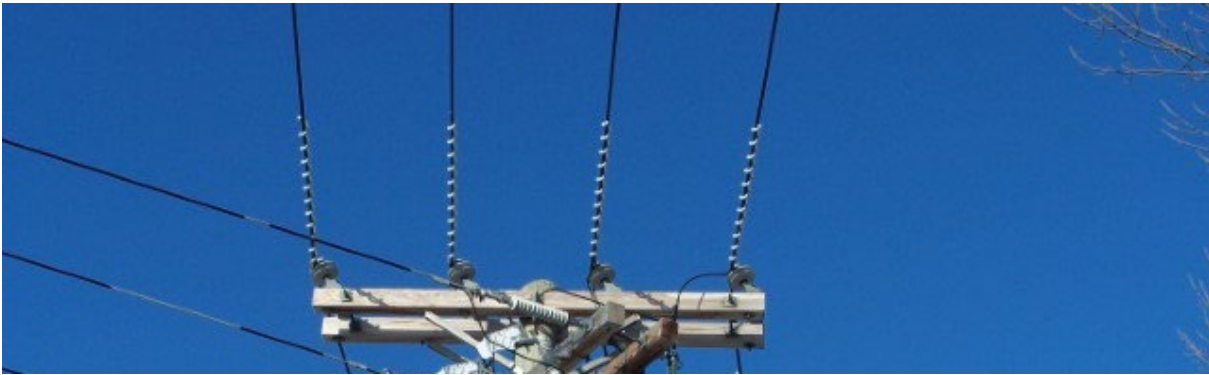
Figure 5.3.G Covered conductor ("tree wire")
